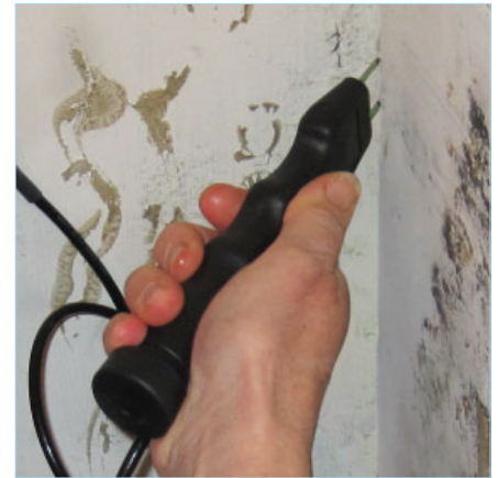
For all areas in the building envelope where the meter pins cannot reach or the display cannot be read. Detect moisture where it hides!
